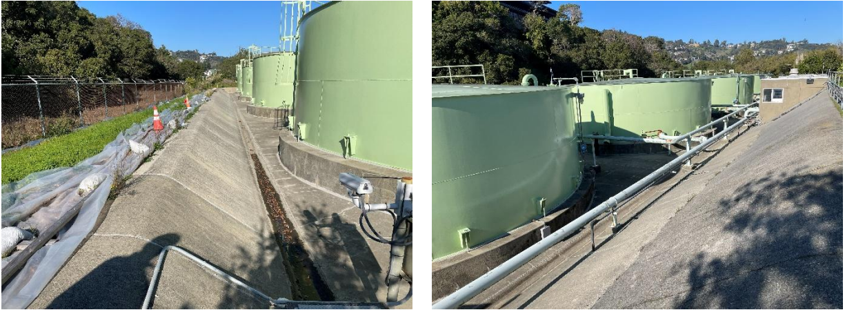
Figure 9. North views of Fuel Tanks, west side (left) and east side and Pump Station (right)
