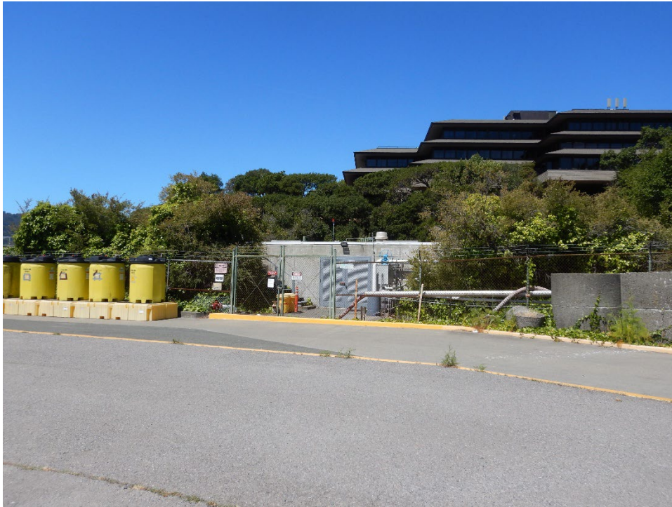
Photograph 11: Fuel tank and pump area, facing southwest.
