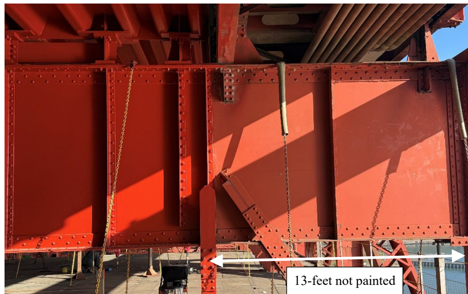
Figure 3 – Example of 13-foot Long Section of Floorbeam Not Painted in Span 4
