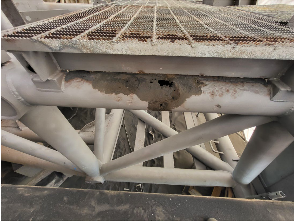
Figure 3-Extent of steel deterioration revealed after steel surface blasting and cleaning operations
