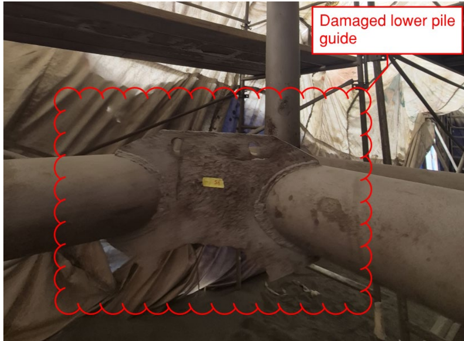
Figure 5-Unforeseen damage to lower pile guide bracket due to its location at the water line
