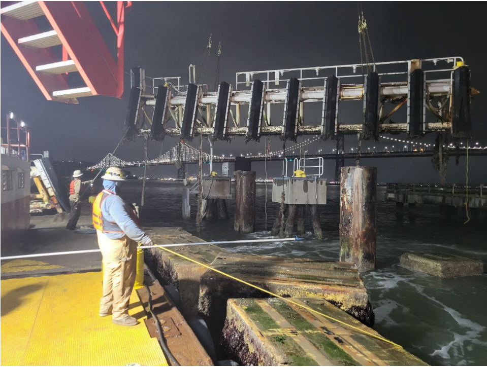
Figure 2-East Camel structure removed from guide piles by crane with polystyrene pontoons disconnected
