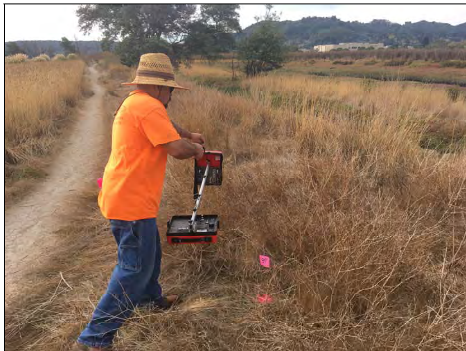
Photograph 4: View of utility locator scanning for subsurface utilities at a proposed soil boring location in sample grid cell B9, looking south. October, 2018.
